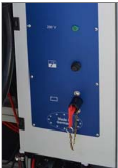
Fig. 1 17 Battery main switch
