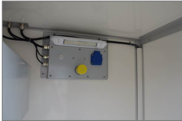
Fig. 1 126 Vacuum cleaner connection in additional chamber
