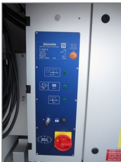
Fig. 1 16 Emergency shutdown switch
