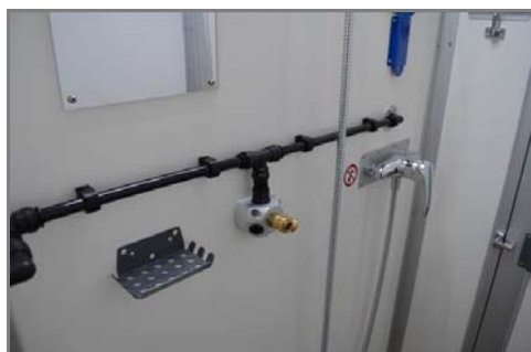
Fig. 1 125 Compressed air supply
