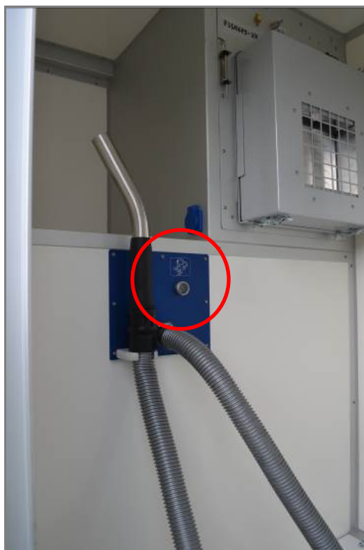
Fig. 1 12 Push-button for activating the vacuum cleaner (red circle)
